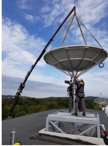
Figure 2.9: Picture from the installation of the TSRS 2.0 antenna system in Basovizza (OAT), Trieste, Italy.
